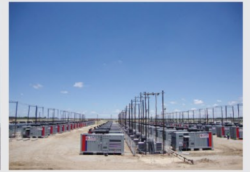
Botswana 70MW diesel power plant ↑
